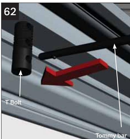
62 From the inside of the conservatory insert the snap off tommy bar into the T bolt
